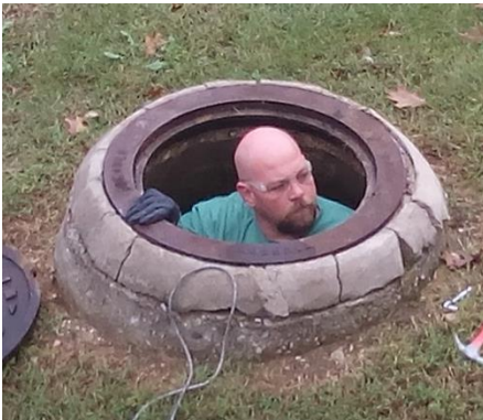
Before--Note the cracks around the lip of the manhole
